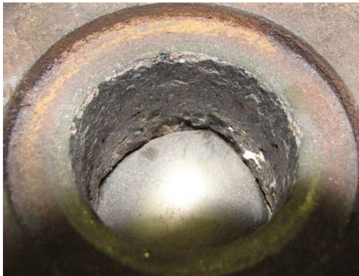
Figure 47—Rupture Disk Holder Subjected to Excessive Corrosion
