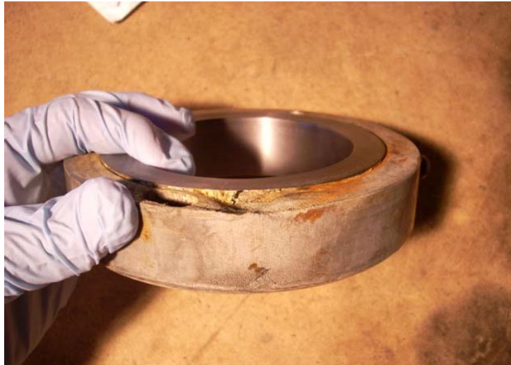
Figure 49—Rupture Disk Holder Corrosion Due to Leakage
